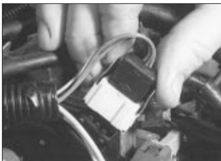
12.2a Disconnect wiring connectors from throttle potentiometer . . .
